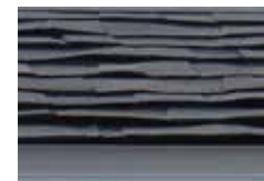
Cupping in shingles without SureNail® Technology
